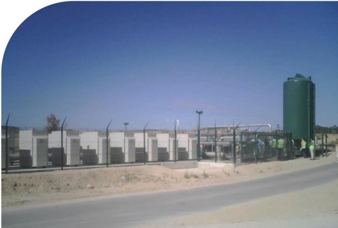
Eighteen C65 microturbines running on methane gas generate power and heat at La Ciotat Landfill in France.
